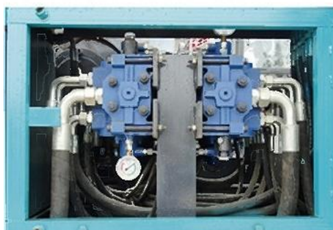
Hydraulic distribution valve
