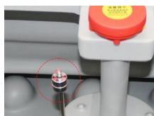
Large-opening recovery tank Water level sensor
