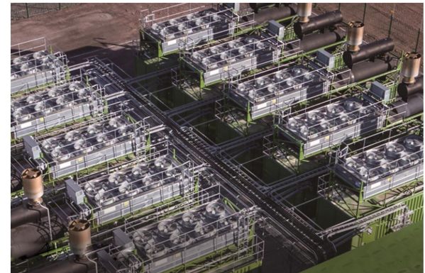
Gas generator power plant
