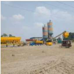
Wet Mix Macadam Plant / CTSB Plant
