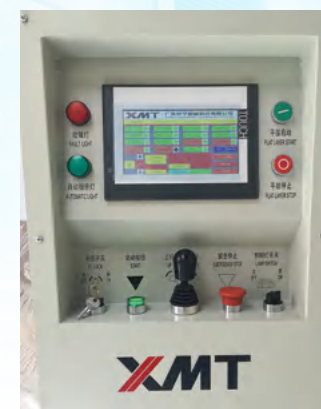
Control panel 操作盆
