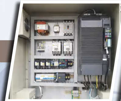
VFC box on the top of cage 笼顶电控箱
