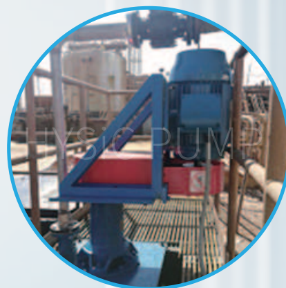
Copper Mine project in Chile
