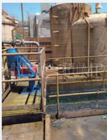
Copper Mine project in Chile
