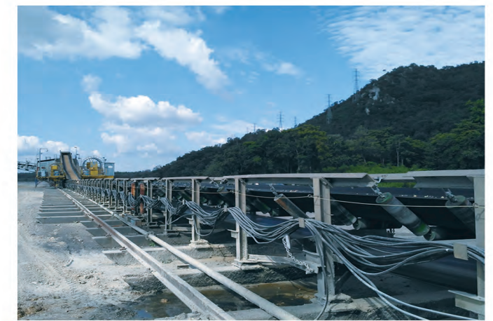
▲ 泰国客户电厂皮带机项目 Belt conveyors system of Thailand power plant
