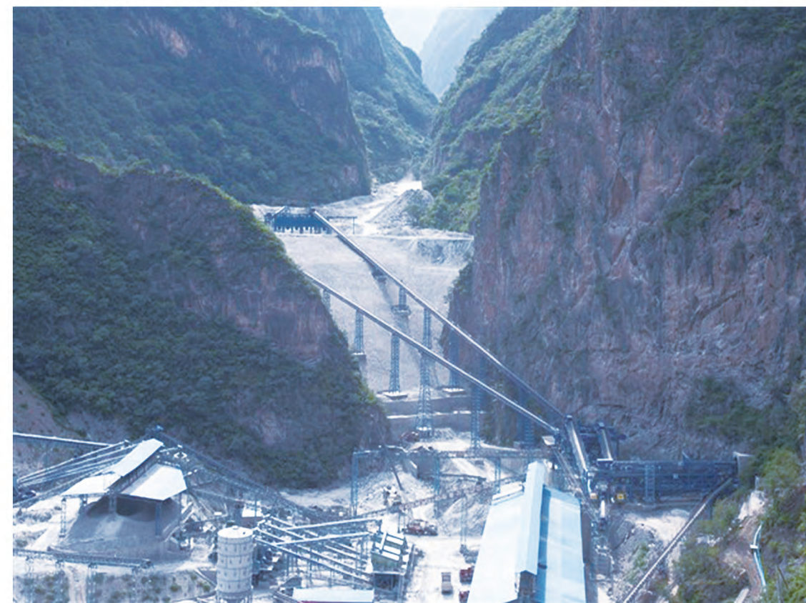
锦屏水电站带式输送机项目 Belt conveyor idlers of Jinping hydropower station
