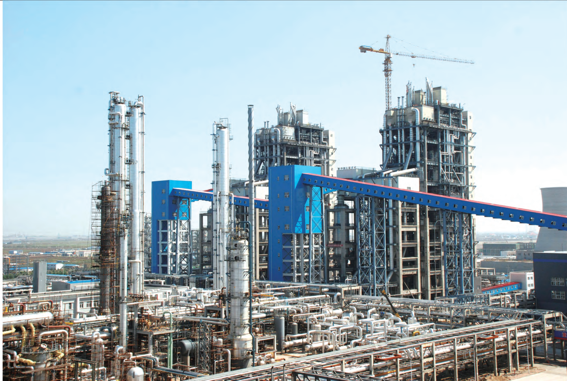
▲ 天津渤化永利化工输煤皮带输送机项目 Belt conveyors system of Tianjin YongLi Chemical Industry
