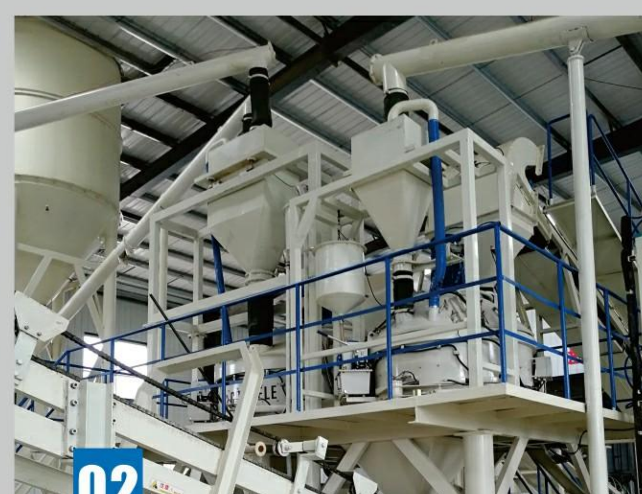
02 Materials mixing system
