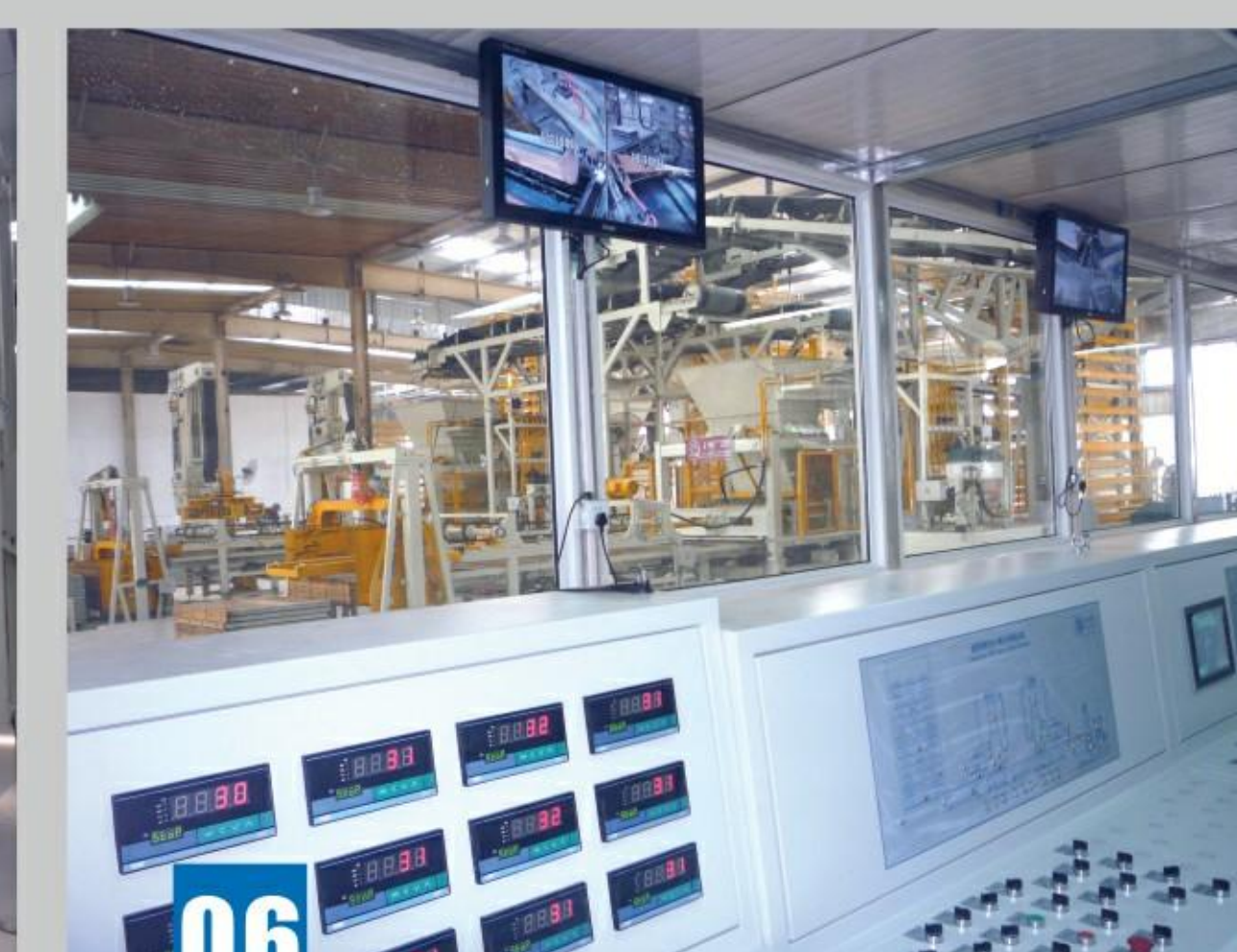
06 PLC control system of the production line
