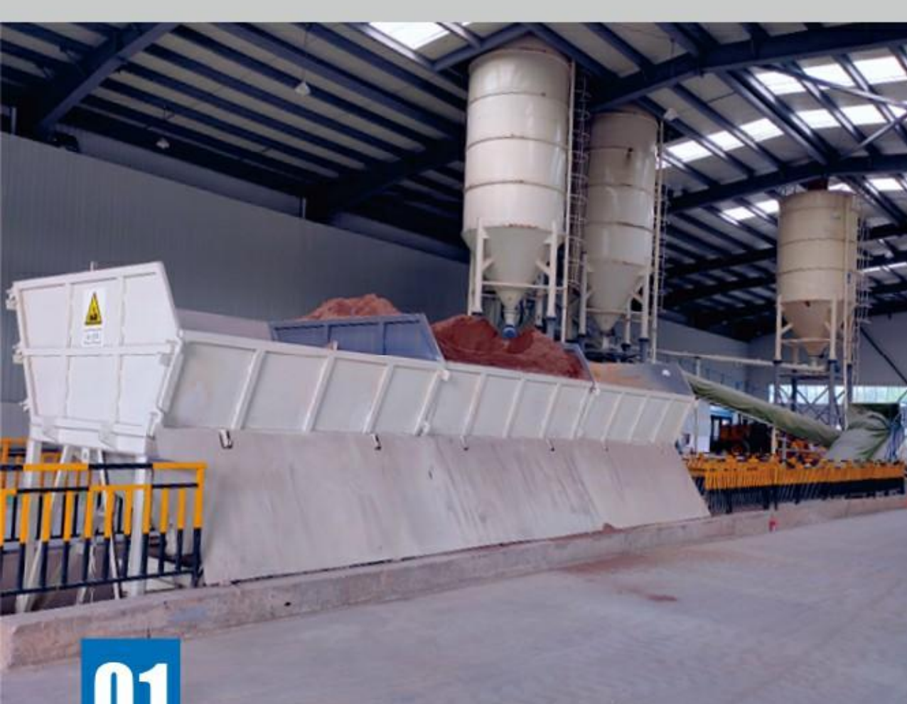
01 Materials batching system
