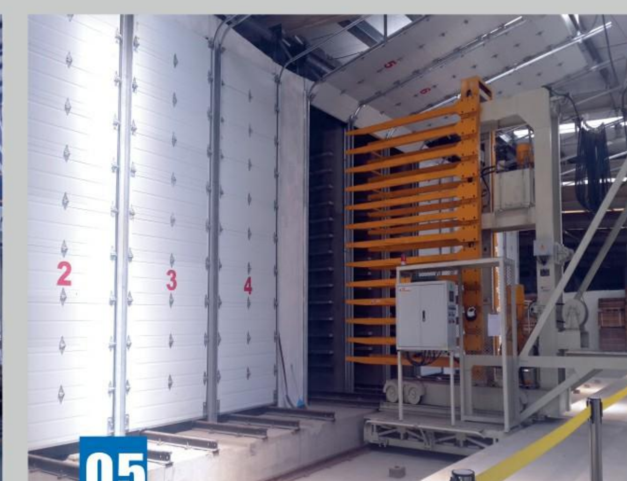
05 Kiln car transferring system
