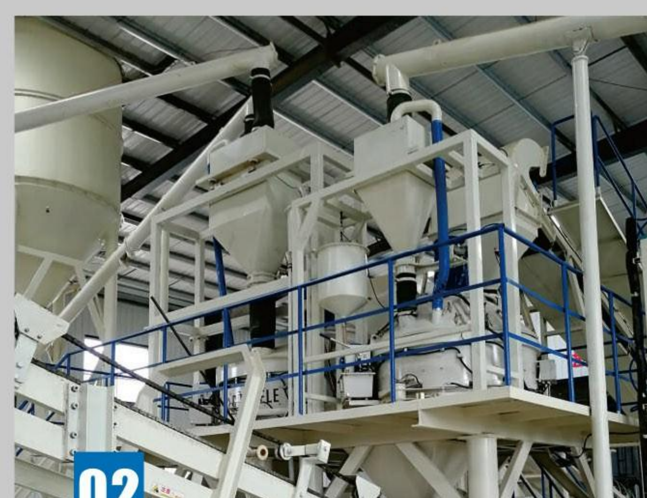
02 物料搅拌系统 Materials mixing system
