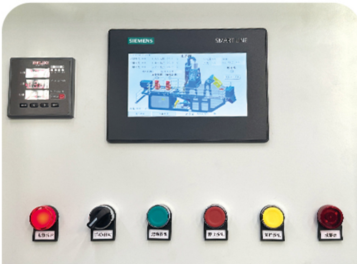
② PLC Automated Controller
