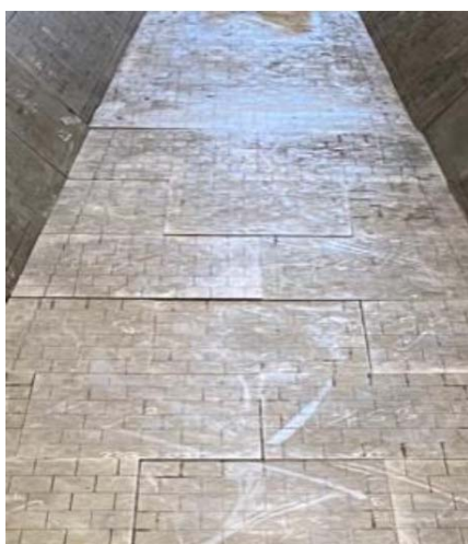
Liners for transfer Chute
