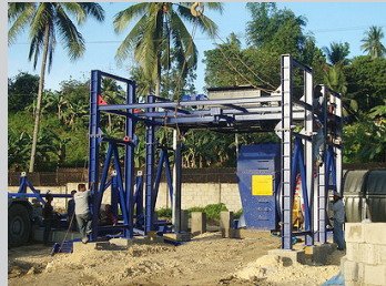
Support structure & mixer modules
