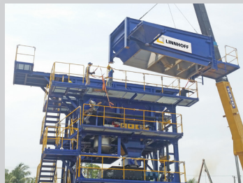
Hot Mineral Bins & Recuperated Filler Silo modules
