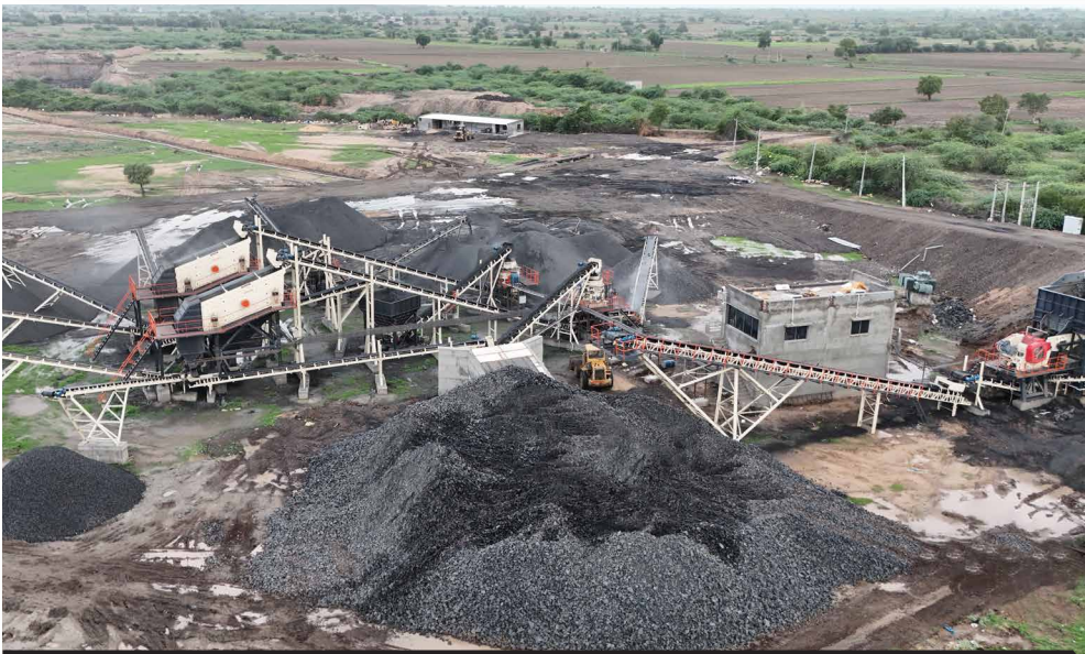
250 TPH - 3 STAGE C&S PLANT WITH WASHING SYSTEM
