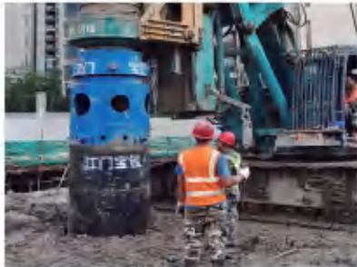
珠海斗门招商依云华府房建桩项目 Zhuhai Doumen Merchant Evian Huafu House Building Pile Project
