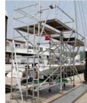
Special tower for yacht maintenance
