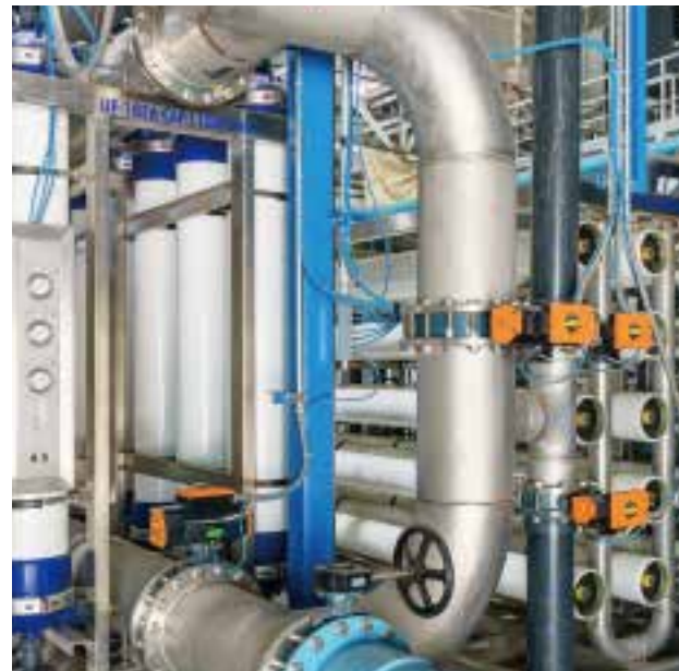
供水系统 Water supply system
