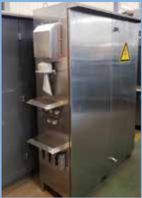
变频控制电控柜 Inverter controlled panel (VFD)
