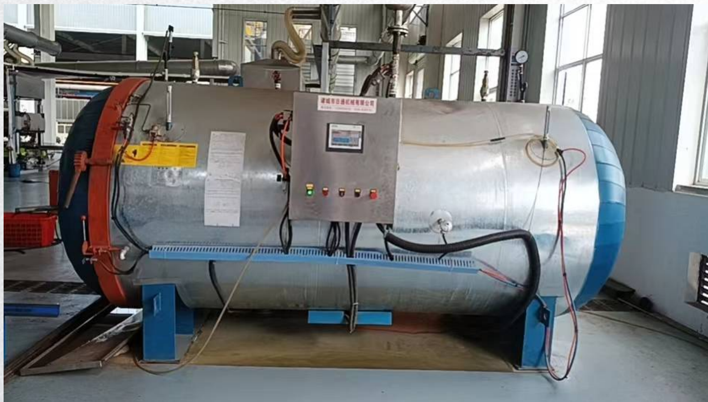
胶管蒸汽硫化罐
