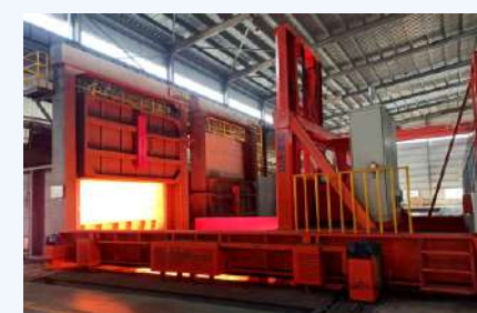
热处理设备 Heat treatment equipment
