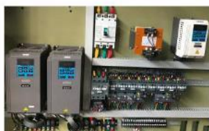
控制柜 Control cabinet
