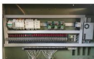
控制柜 Control cabinet
