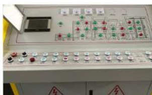
控制柜 Control cabinet
