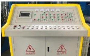
控制柜 Control cabinet
