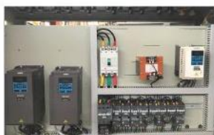
控制柜 Control cabinet inside
