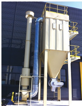
隆翠汽车木工区域除尘 Longtree Automobile Woodworking Dedusting Plant, Zhejiang, China
