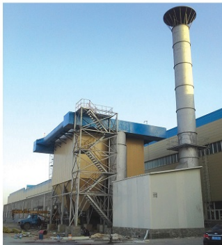
常铝股份熔铸线除尘器 Casting Dust Collector, Fujian, China
