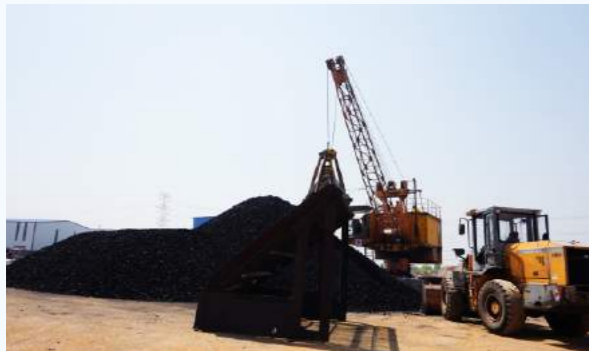
溧阳客户现场图 Customer Scene in Liyang
