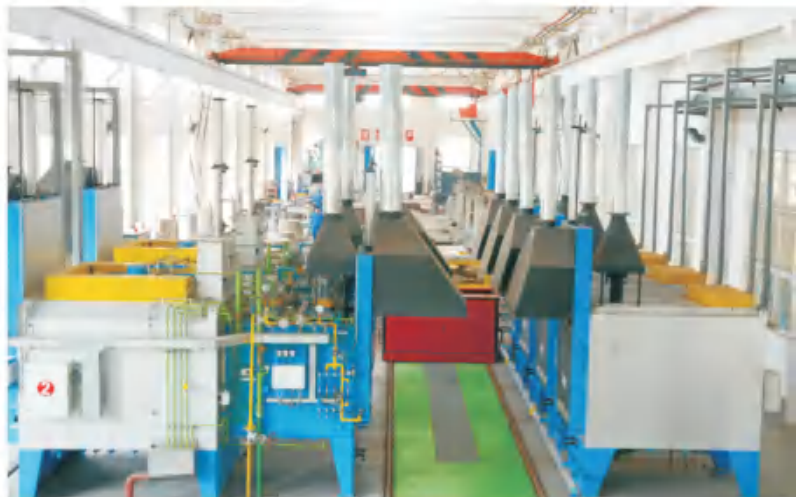
▲ Italy Ji Aifei produced heat treatment production line
