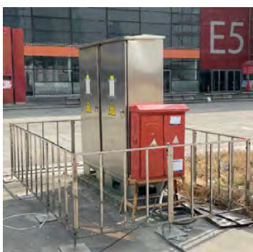
电箱 Power Supply Box
