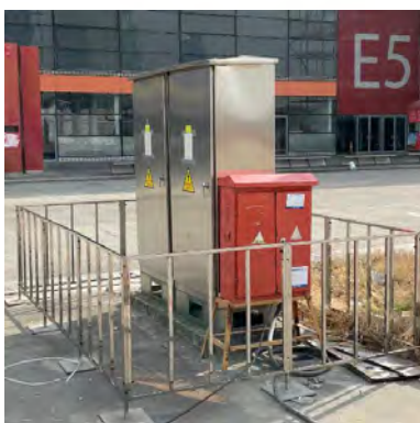
电箱 Power Supply Box
